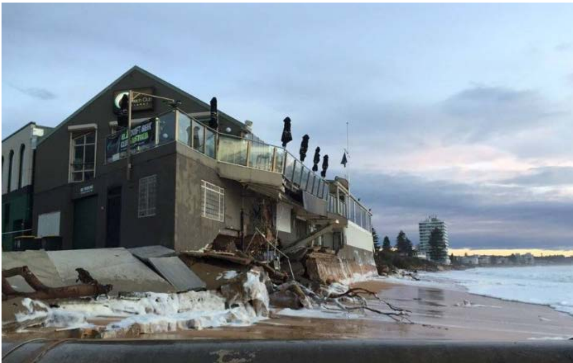
Collaroy Surf Life Saving Club - damage from recent Sydney Storms
